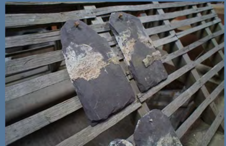
Above: Traditional pegged-slate roofing which lasts centuries and can easily be repaired.
